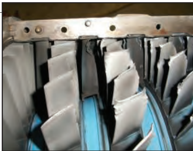
FIGURE 2. Axial compressors are very vulnerable to damage from surges. This photo depicts the type of blade damage that can be expected as a result of a surge event in an axial compressor
